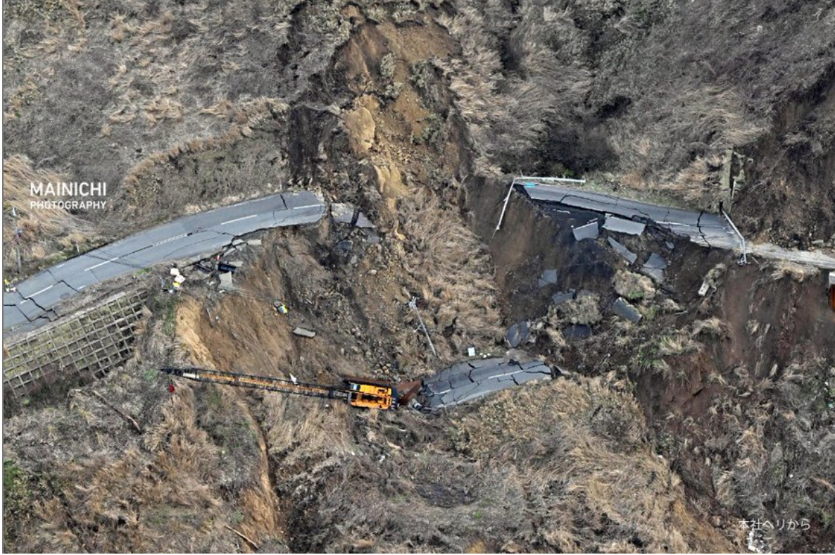
Figure 2: Road destroyed by landslide due to earthquake [2]
